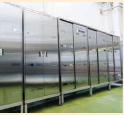
Securing spaces beneath the racks
