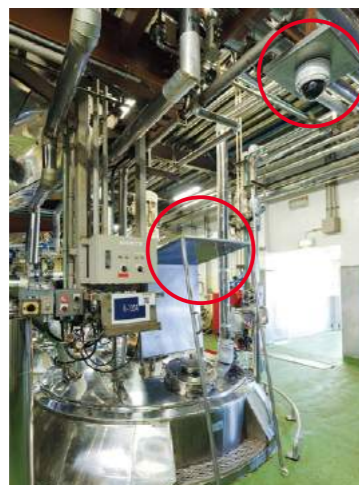
Monitor cameras are installed at ingredient input ports.
